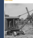
Object Type: Photograph Construction work going on at 63rd Street and State Line, with a crane being prepared for ground for street paving.
